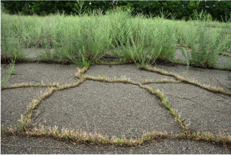
Urban vegetation takes hold in cracks in a neglected swath of asphalt pavement.
